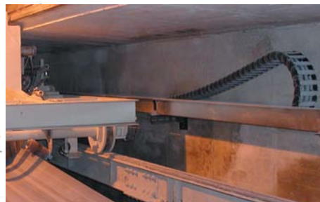
Ventilation machine in a lime plant
