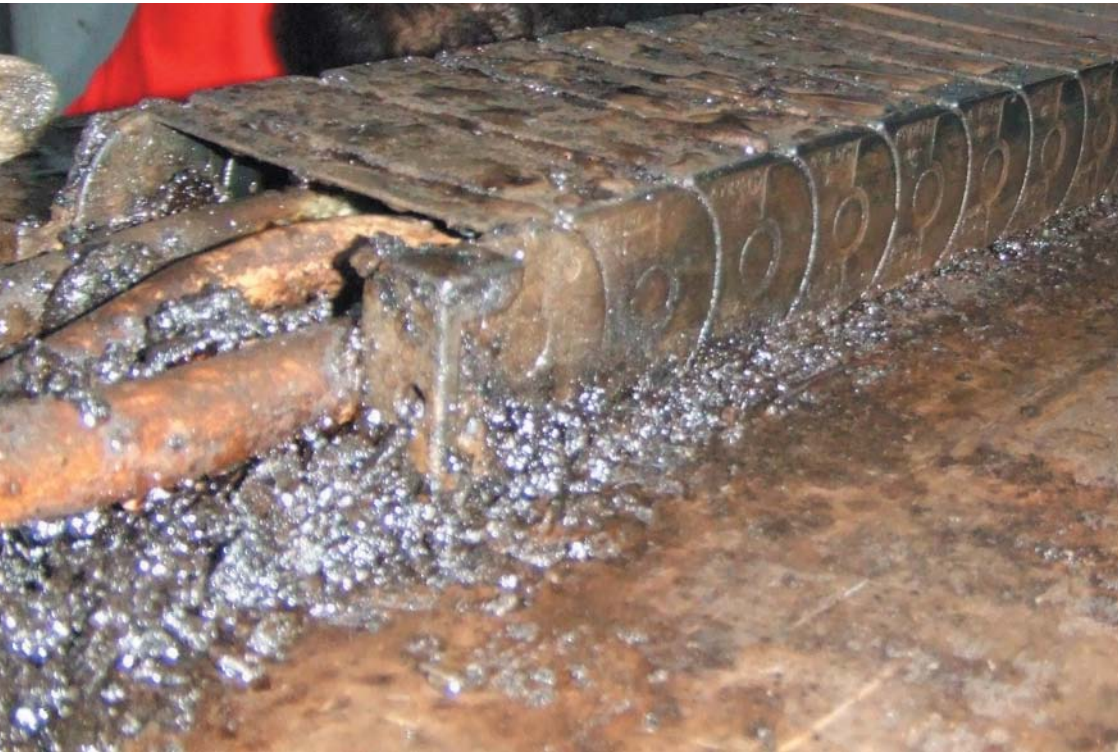
Debris from construction materials creates an extremely hazardous environment.
