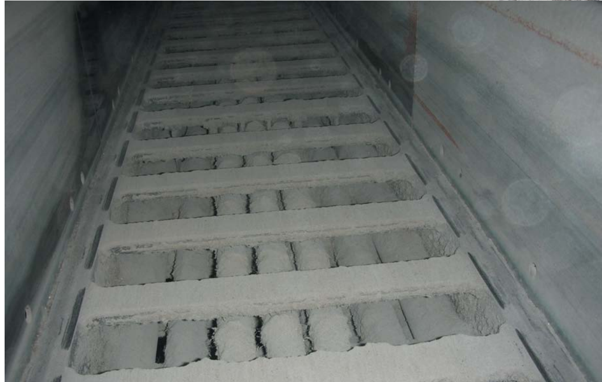
Refuse incinerator plant encounters caustic substances and still performs flawlessly.
