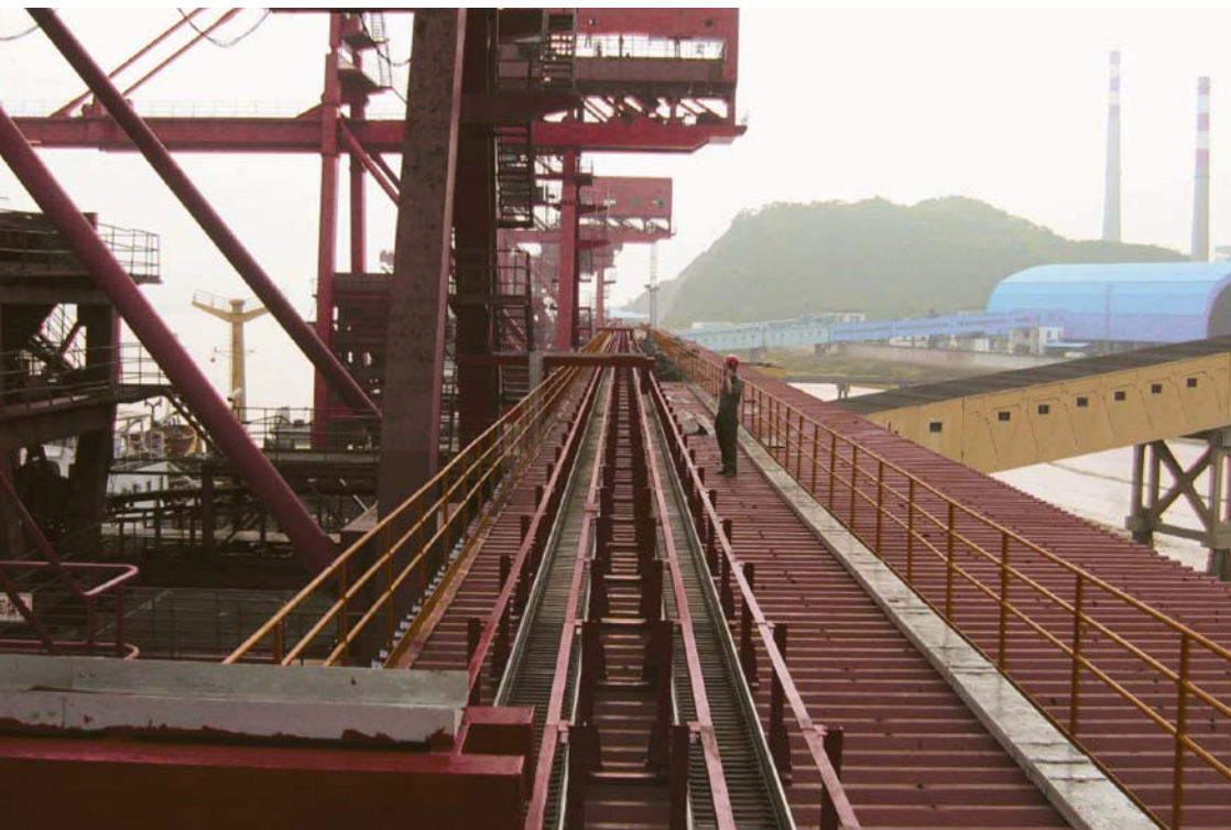
A Rol-E-Chain System with a 190 m travel length is installed in a coal burning power plant.
