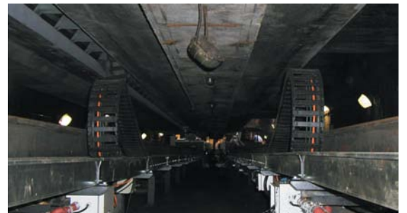
Ventilation system in underground storage at a power plant
