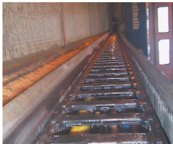
Energy Chain® with Chainflex® in a truck washing facility with fine road-dust and gravel/mud debris
